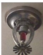
Sprinkler system function properly maintained
