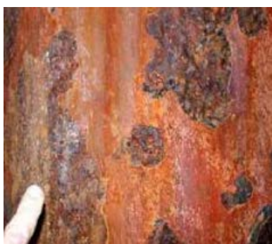
PSC Detainable Deficiency
