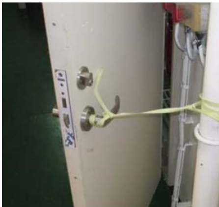
PSC Detainable Deficiency
