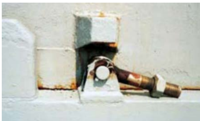
PSC Detainable Deficiency
